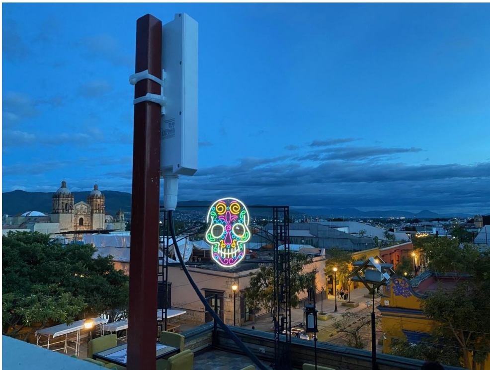
(Hotspot deployment in Oaxaca, Mexico)
