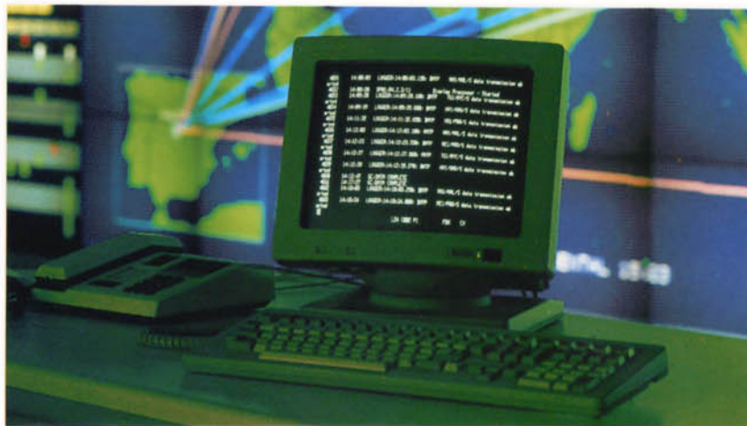
Dynamic Network Management Centre at the Alcobendas (Madrid) international exchange.
