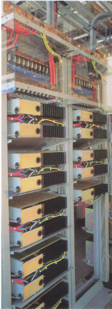
Detail of the mobile telephony installations in the Cartuja-Sevilla Exchange.
