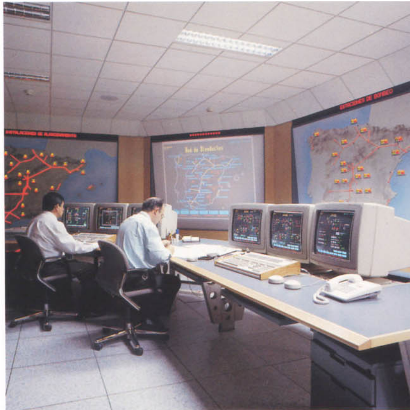
Telecommunications control room at Campsa headquarters, Madrid.
