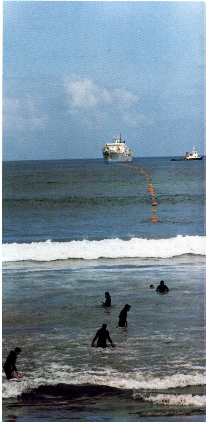
Laying of the OPTICAN optical fibre submarine cable between Tenerife and Gran Canaria.
