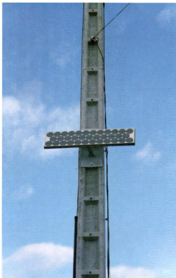
Detail of rural telephony equipment.
